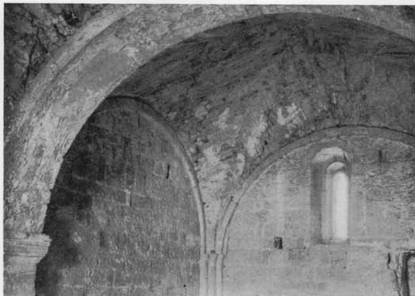
Fig. 3. The groined cross-vault in Italy, built without solid centering, on skeleton diagonals. Vault, in crypt, S. Maria del Solario, Brescia. Dating about 1120.
